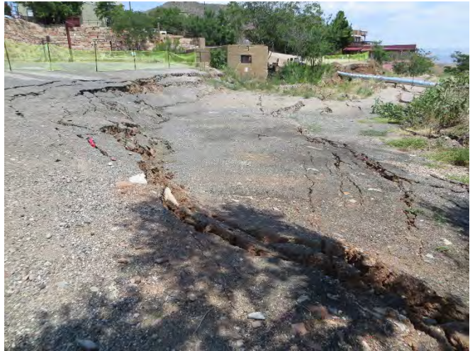
Figure 70 Photo of Jerome Landslide Related Damage
